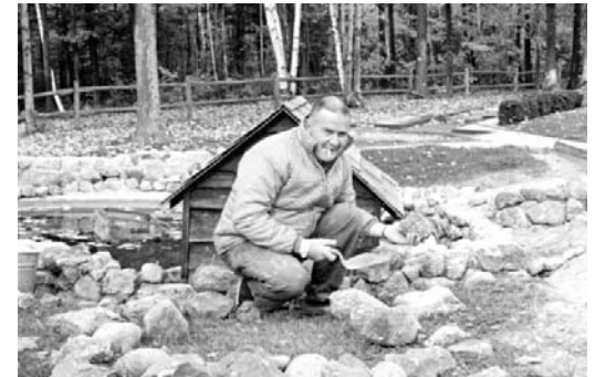
Master stone mason John Lawton building the wall next to the water wheel. From the mid 1960's up until John's death in 2003, he constructed 599 feet of walls on the mini-golf!
