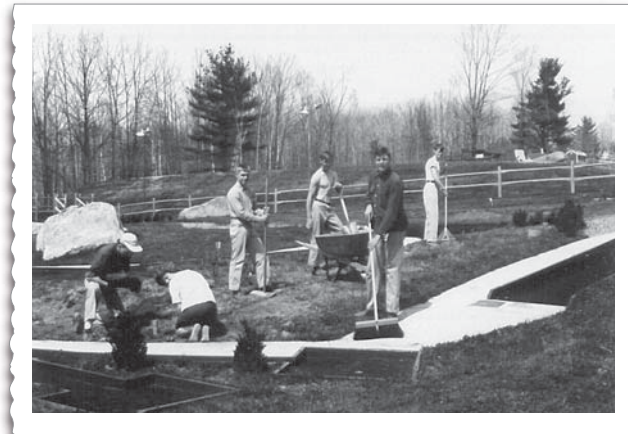
By mid-July, 1964, construction was nearing completion. Several boys from the state school were brought in to help.
